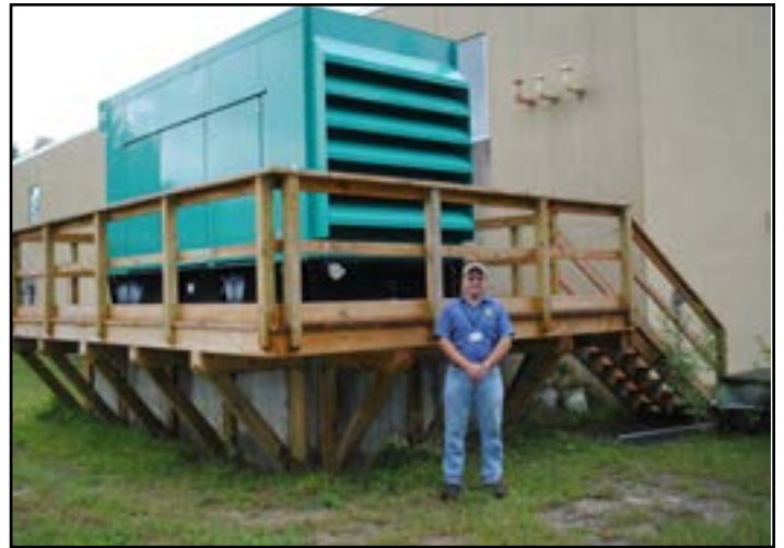
Somerset, NH drinking water facility's generator was elevated after two flooding events
